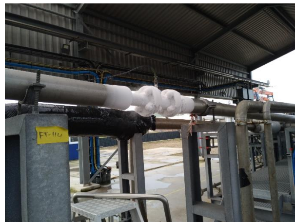
Figure 1: TrigasDM turbine LH2 flow meter installed in VSL’s LNG calibration and test facility [11].
