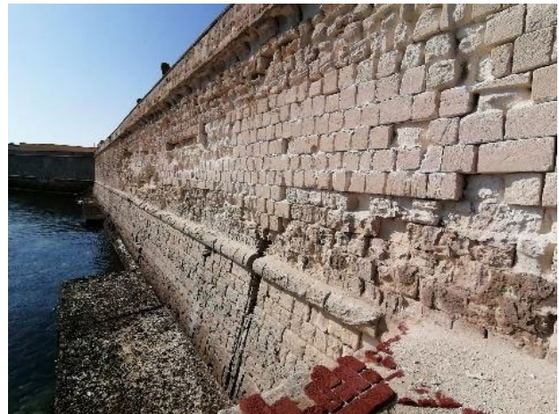
Fig. 2. Stabilimento Florio in Favignana (TP). Deterioration with alveolation and patina of the external wall surface | © G. Cacciaguerra, CNR ISPC.
