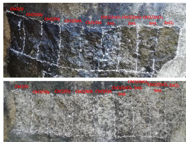
Fig. 4. After DESs application (above) and four months after application (below) on an effusive magmatic rock at the University of Calabria.
