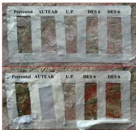
Fig. 3. Before application of DES 6 (above) and after application (below) during conservative treatment of wall painting in Motta San Giovanni (Reggio Calabria).
