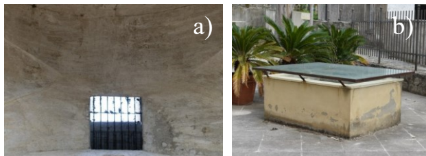
Fig. 4a. Skylight hollow viewed from the inside of the church; Fig. 4b. Skylight viewed from the outside of the church.
