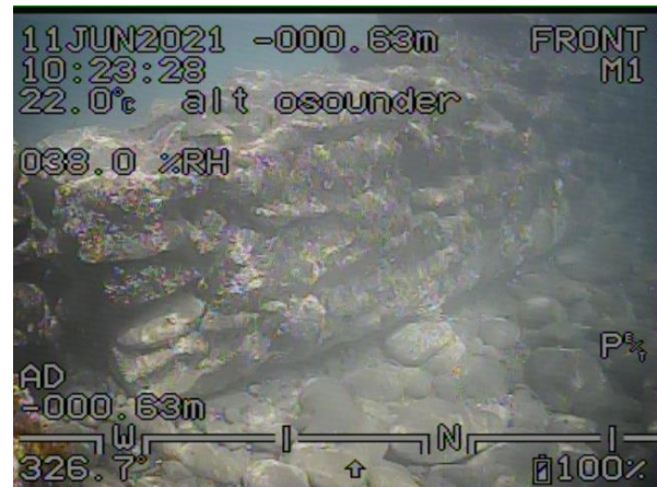
Fig. 4. Scouring effect in a wall of the structure
