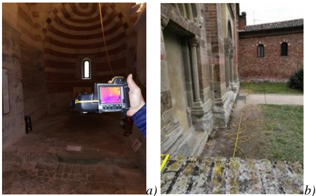
Fig. 3. Example photographic documentation of the geophysical survey methodologies: a) Geoelectric and b) IR thermography carried out for the diagnostic study of the Vezzolano Rectory.
