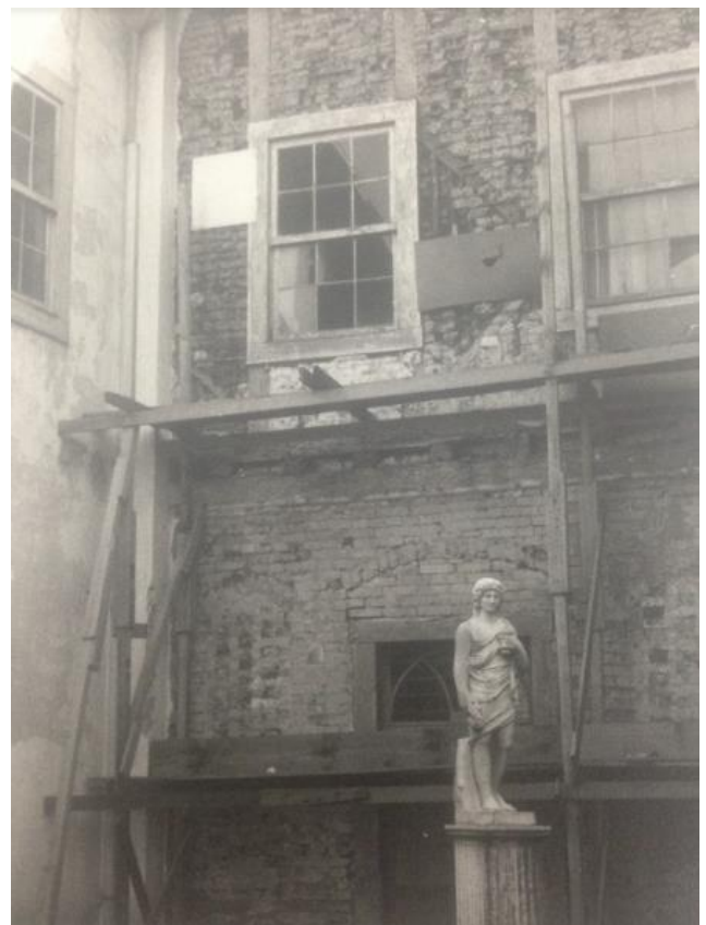
Fig.3. Photograph of the MRCI rear façade and the architectural restoration works from the 1970s.
