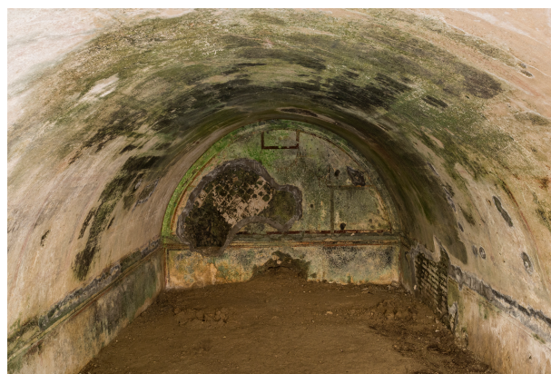
Figure 1 – Detail of the room SB-E0-R07. It is possible to notice the massive presence of biodeteriogens in particular on back wall and on the ceiling.
