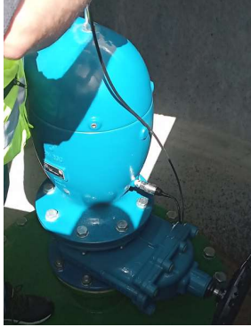
Figure 11: Connection of the pressure transducer to one of the conduct's air valve
